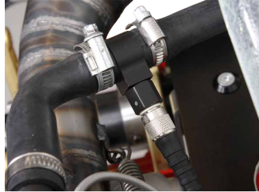
T-junction mounted in the cooling water hose with a temperature sensor.
